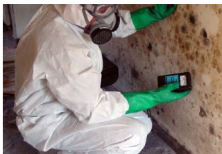
Mold infestations often occur in dark, moist areas without proper air circulation and can quickly spread.
