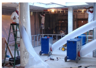
Extensive mold impacts may require significant remediation efforts to repair, but the process is predictable and finite.
